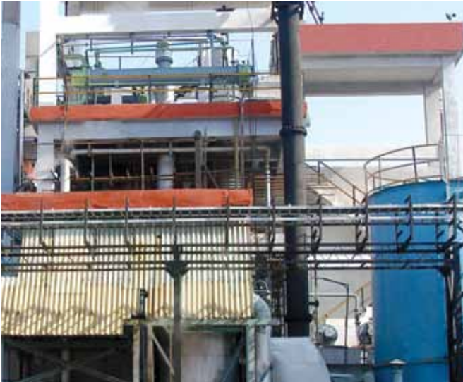
New membrane plant
