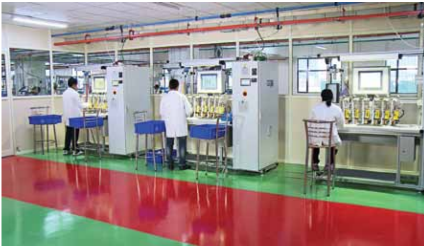
Another view of the switchgear plant
