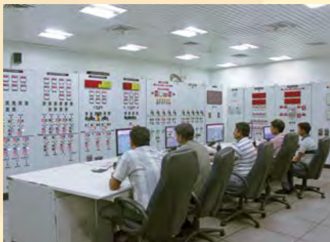
One of the turbines and control rooms of the new 55 MW power plant
