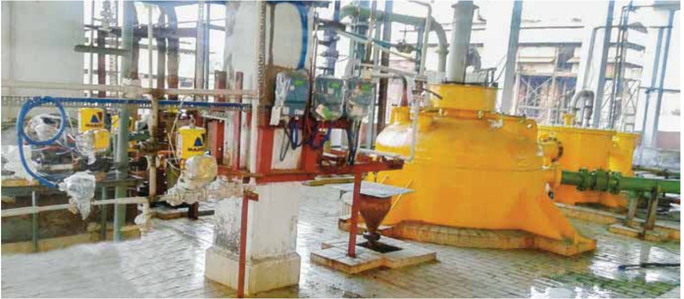
The modified chlorine dioxide plant
